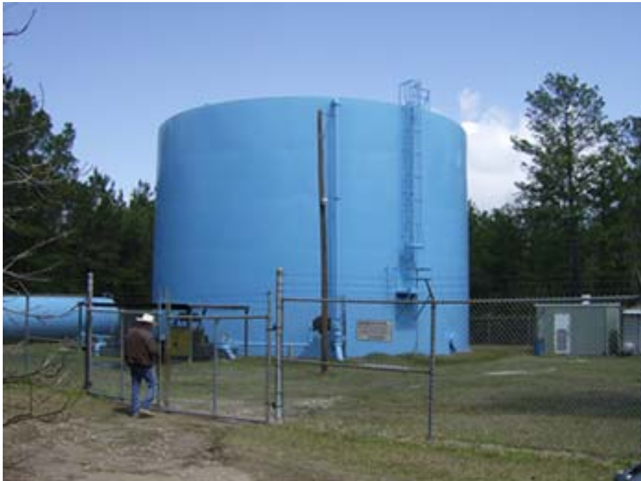
Waterwood MUD Storage Tank
